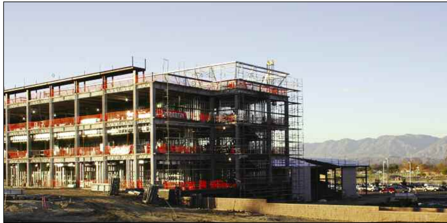
In the photo above, taken Thursday, December 14, the steel girder outline of the Centennial Complex is nearly complete.
