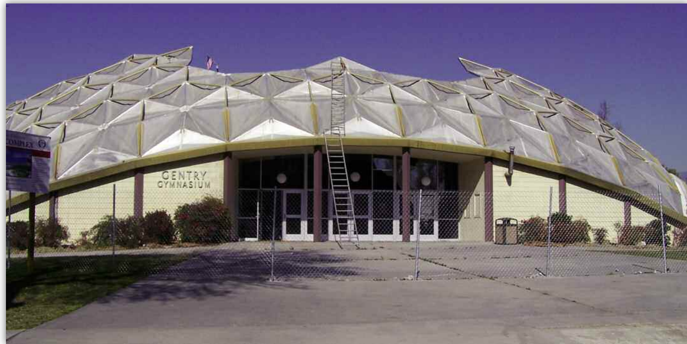
Mount St. Helens-like, the top of Gentry Gymnasium has already disappeared in this photo taken on February 10, 2006. For a current real-time view of dismantling progress check the Internet live-cam site at < www.llu.edu/centennial/complex/construction.html >.
