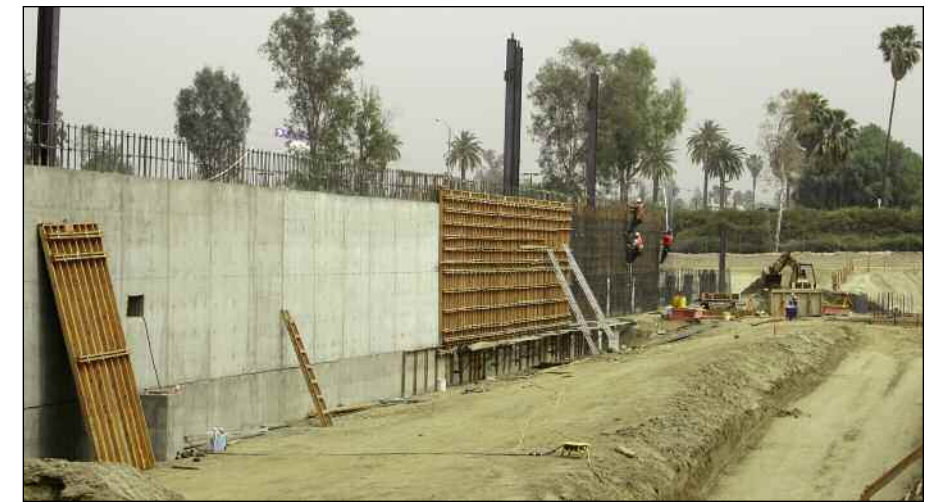
Construction has now begun on the Centennial Complex. This picture, taken March 20, shows the beginnings of the south wall.
