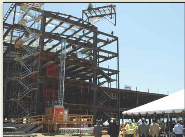
A crowd watches Thursday, May 21, as a construction crane hoists the last piece of steel beam for the new Loma Linda University Medical Center–Murrieta. ▲
