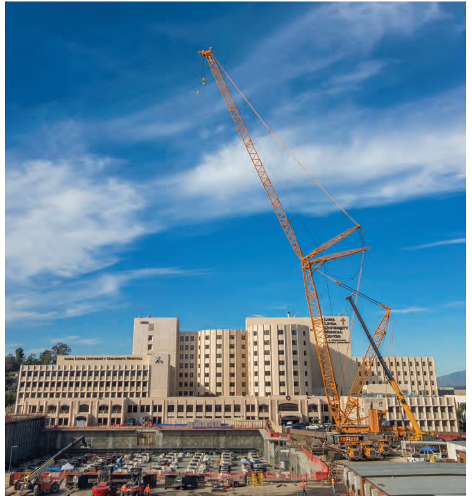
Massive cranes will be used to place the steel needed for Loma Linda University Health's construction project to build a new adult hospital and expanded Children's Hospital.
